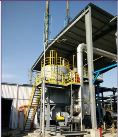
Regenerative Thermal Oxidizer at allnex plant in Fengxian, China
